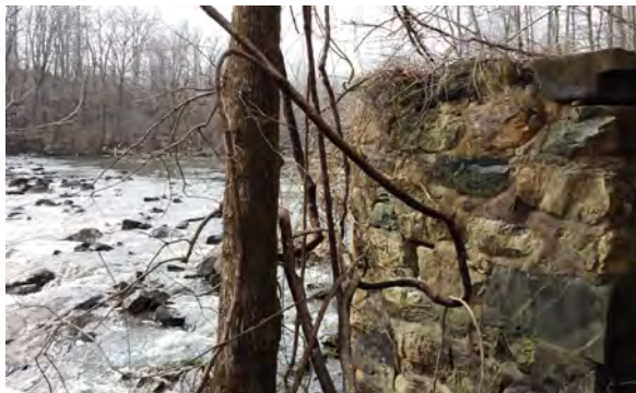
Abutment of the old dam at Carolina Falls as seen from the Haw River Trail. Photo courtesy of Katie Gensel
